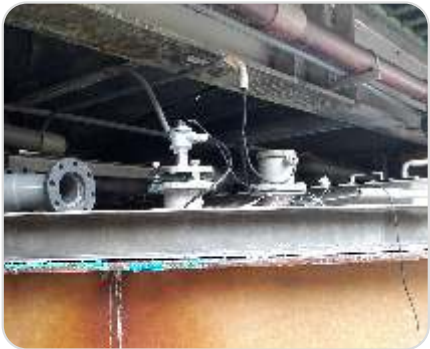
Copper sulfate storage tank
