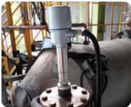
High temperature boiler
